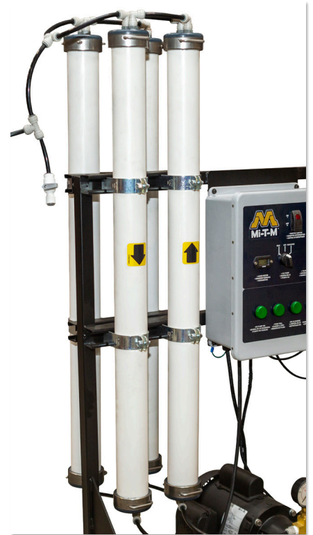
Freshwater reverse osmosis membranes with permeate outlet and sampling port
